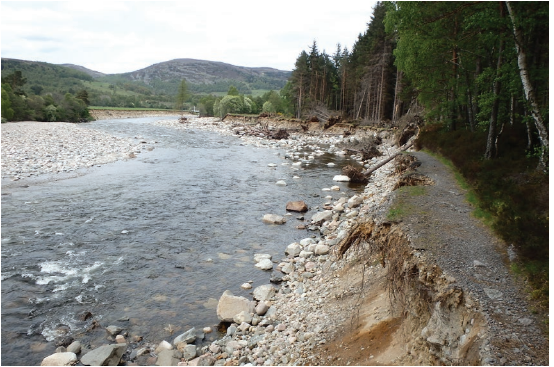
Figure 2. Collapsed bank along the middle reaches of the River Dee
